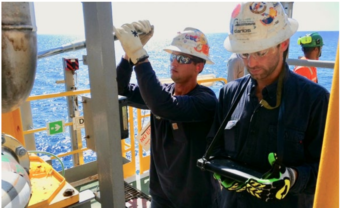
Pipefitters working on a flange on a Shell floating production, storage and offloading facility in the Gulf of Mexico.
